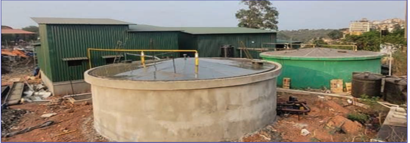
5 TPD Biogas Plant at Taleigao, SBM Project, Goa
