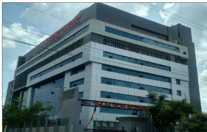
Construction of Super Specialty Hospital at Indore for Ministry of Health & Family Welfare under PMSSY Scheme
