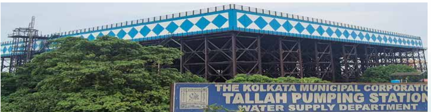
Renewing of 9.0 Mg Capacity Century Old Overhead Balancing Steel Reservoir (Tallah Tank) Under AMRUT for Kolkata Municipal Corporation (KMC)
