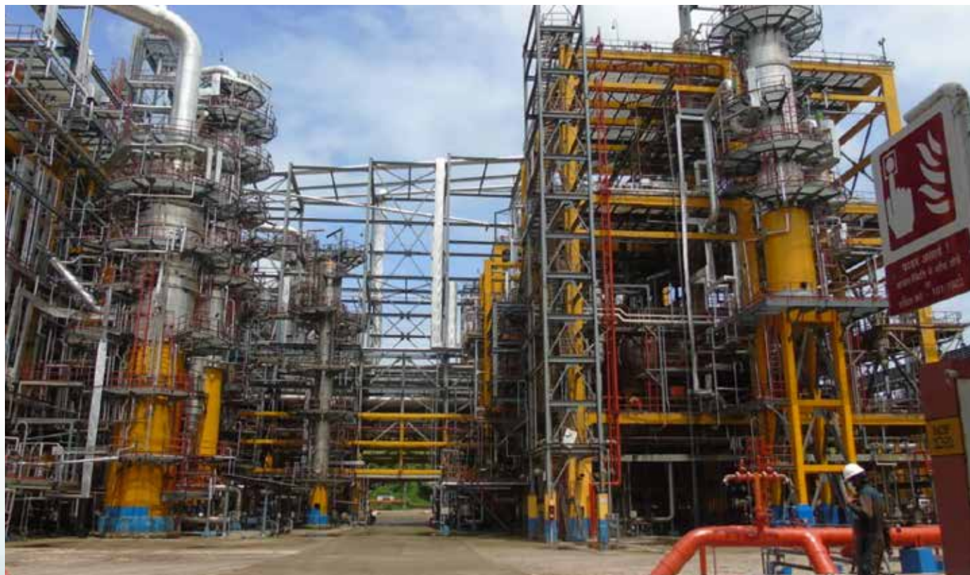
Acrylate Unit at BPLC Kochi Refinery
