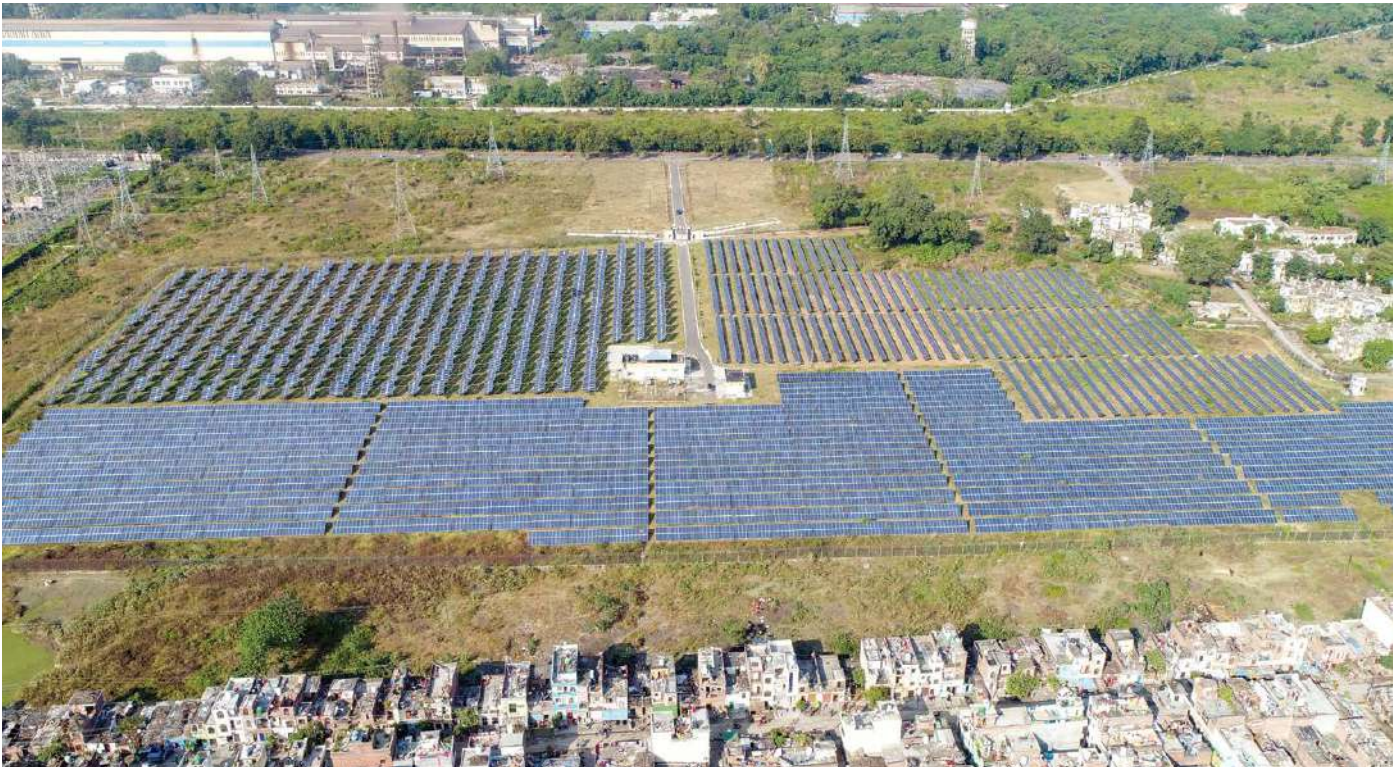
5 MW in-house solar PV installation at BHEL Haridwar for captive power generation
