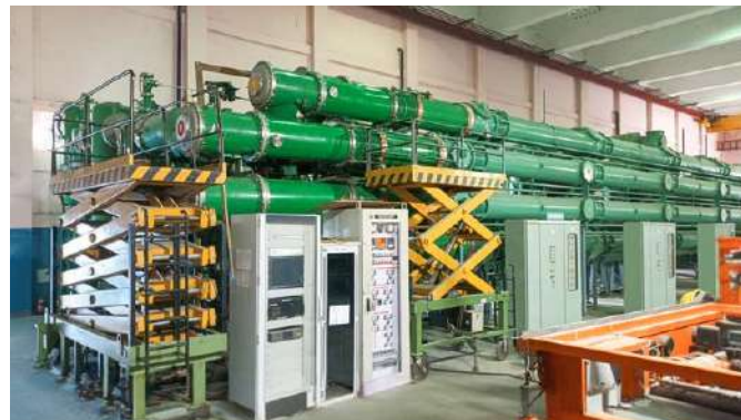
400kV Gas Insulated Switchgear (GIS) bay at Chamera HEP indigenously developed by BHEL under the Aatmanirbhar Bharat initiative
