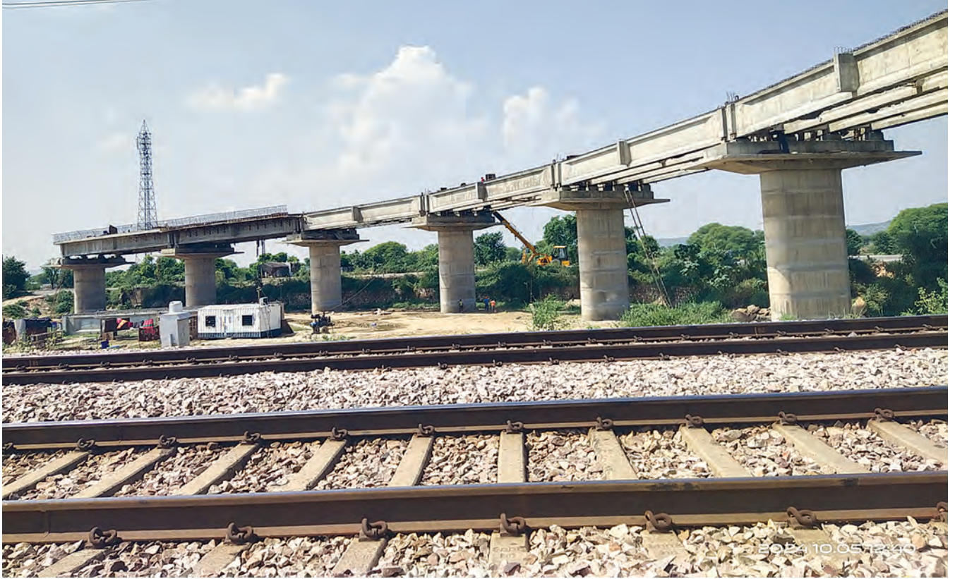
RCC GIRDERS LAUNCHED AT LC NO. 224X - ROB-11 PROJECT ON KOTA-MATHURA SECTION
