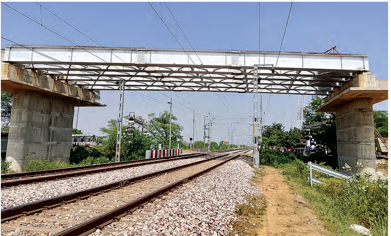
COMPOSITE GIRDER LAUNCHED AT LC NO. 224X - ROB-11 PROJECT ON KOTA-MATHURA SECTION
