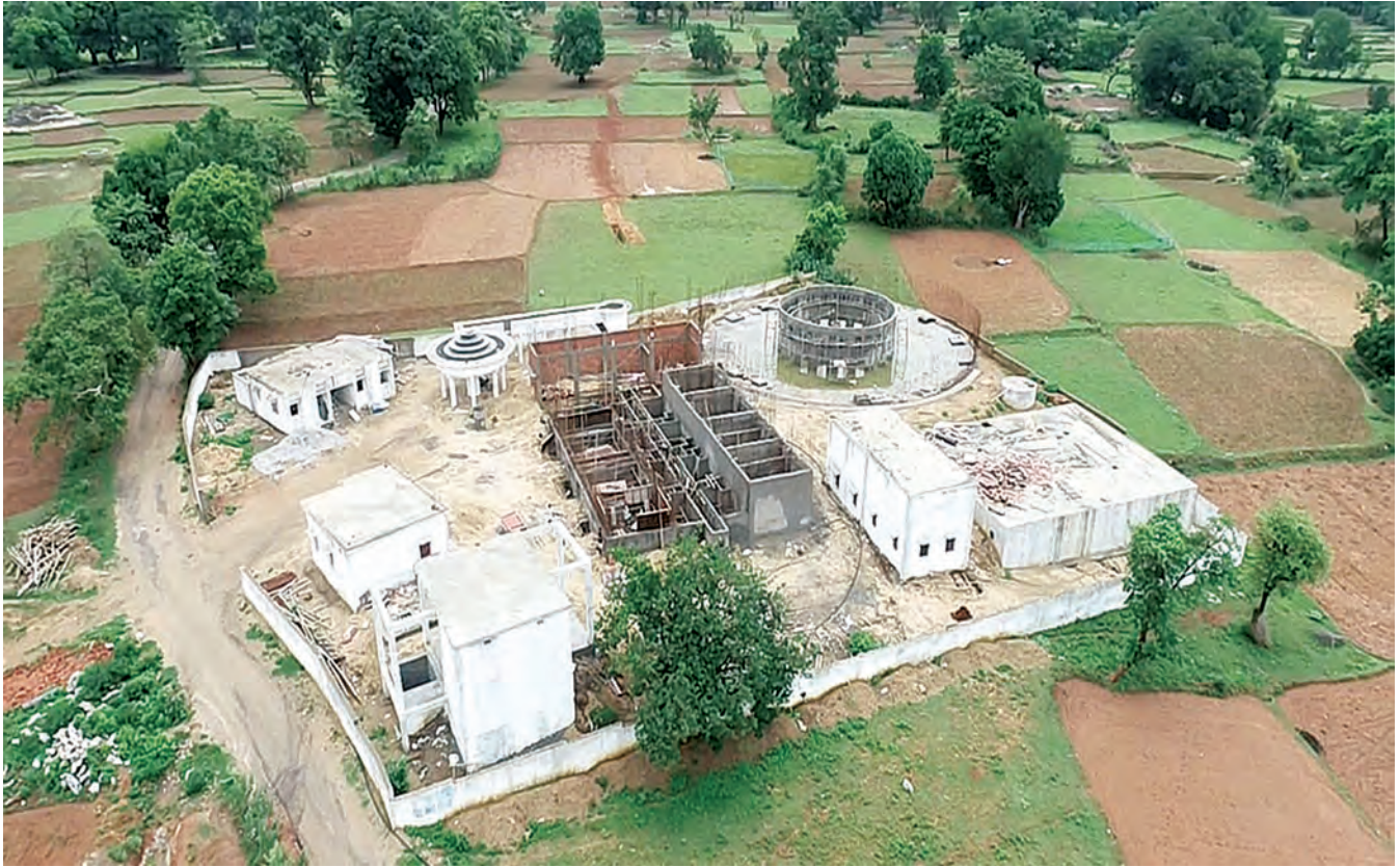
WATER SUPPLY PROJECT SISAI, GUMLA, JHARKHAND- WTP
