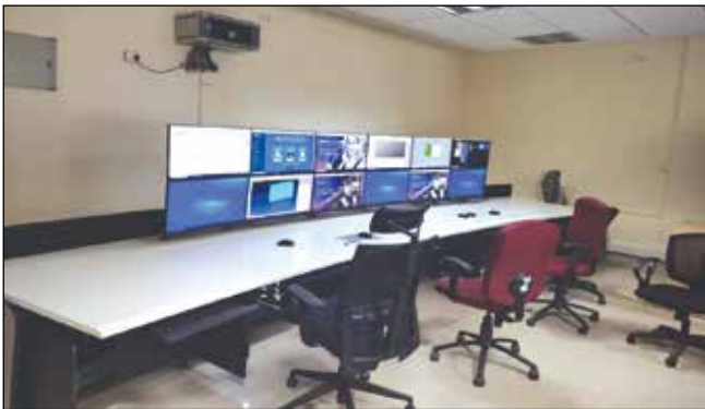
Master control room for smart factory
