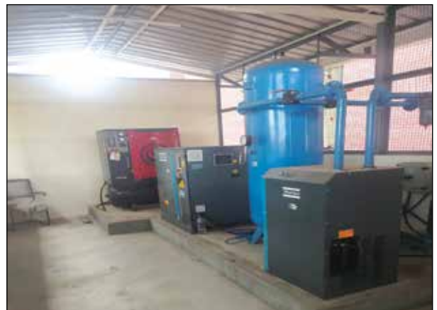
Compressor Room and compressor installed for Workshop
