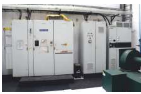
Standby Electric Drive
