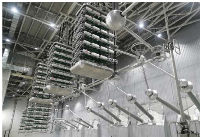
DC Hall of \pm 800 kV, 6000 MW UHVDC link between the Western Region Grid (Raigarh, Chattisgarh) and the Southern Region Grid (Pugalur, Tamil Nadu) successfully implemented by BHEL
