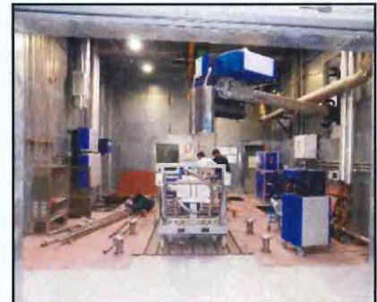
Engine Test Cell
