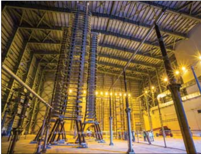
World's first + 800 kV pre-engineered Indoor DC hall at NE-Agra HVDC terminal
