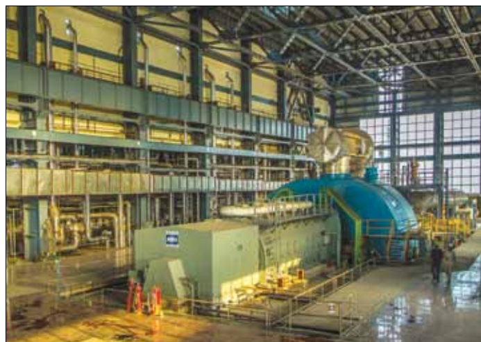
Turbine hall of BHEL's first ever 700 MW supercritical unit at Bellary STPS, Karnataka
