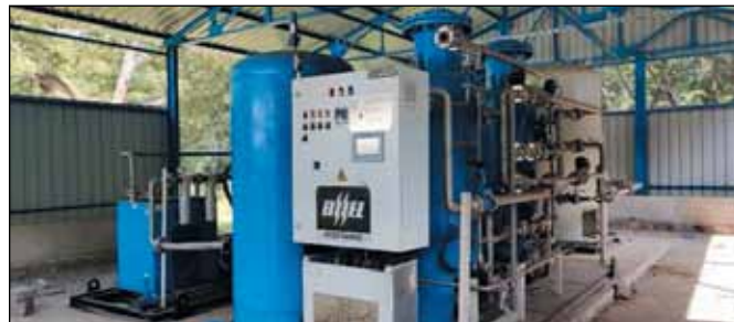
Oxygen Generation Plant at Main Hospital BHEL HPEP, Hyderabad
