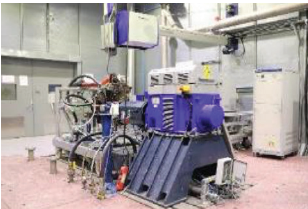
Engine Test Cell
