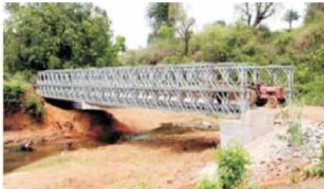
Construction of Bailey Type Unit Bridge at various locations for Government of Odisha
