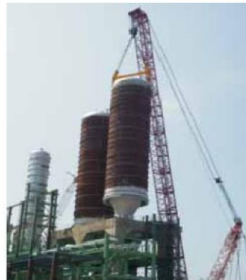
Erection of Two Coke Drums of 575 MT at DCU, CPCL, Chennai Site by Main crane 1250 MT capacity and tailing crane 550 MT
