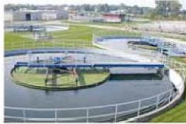
WATER TREATMENT & ALLIED WORKS
