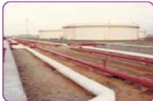
Product Storage Tanks with connecting pipeline at IOCL Kandla
