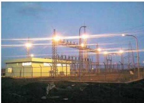
230 kV Substation, Ethiopia
