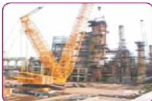
CDU / VDU Revamp at CPCL Manali
