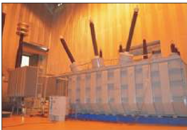
315MVA 400/220/55/33 KV, 3-phase shunt unit of phase shifting transformer under test
