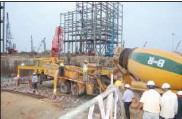
Casting of TG raft power block for 2 x 660 MW Krishnapatanam Thermal Power Project of Thermal Powertek corp India Ltd. by B & R.
