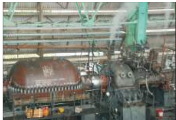
2MCL1007 Compressor for MRPL at BHEL Hyderabad
