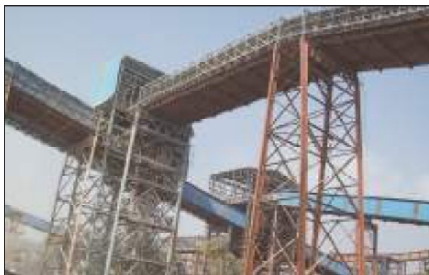
Conveyor System at New Ore Bedding & Bleding Plant Rourkela Steel Plant, HEC
