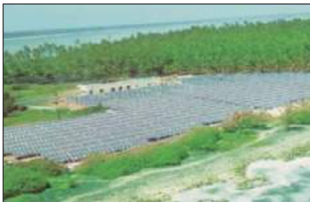
Country's largest Diesel Grid – Interactive Solar Power Plant of 760 kWp capacity, commissioned by BHEL at Lakshwadeep
