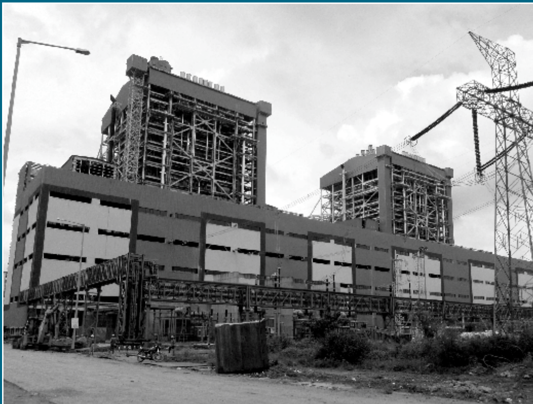
Main Power House Unit 1 & 2 at NTPC Gadawara 2X800 MW STPP
