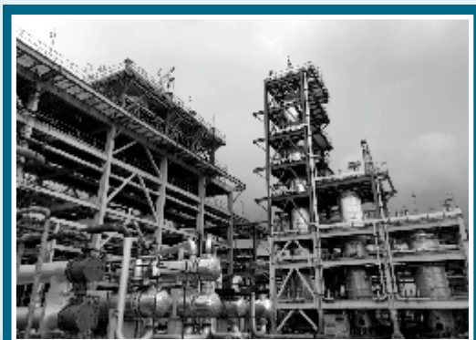
Civil, Structural and UG Piping works for New Process Units at IOCL Gujarat Refinery at Vadodara BS VI Project
