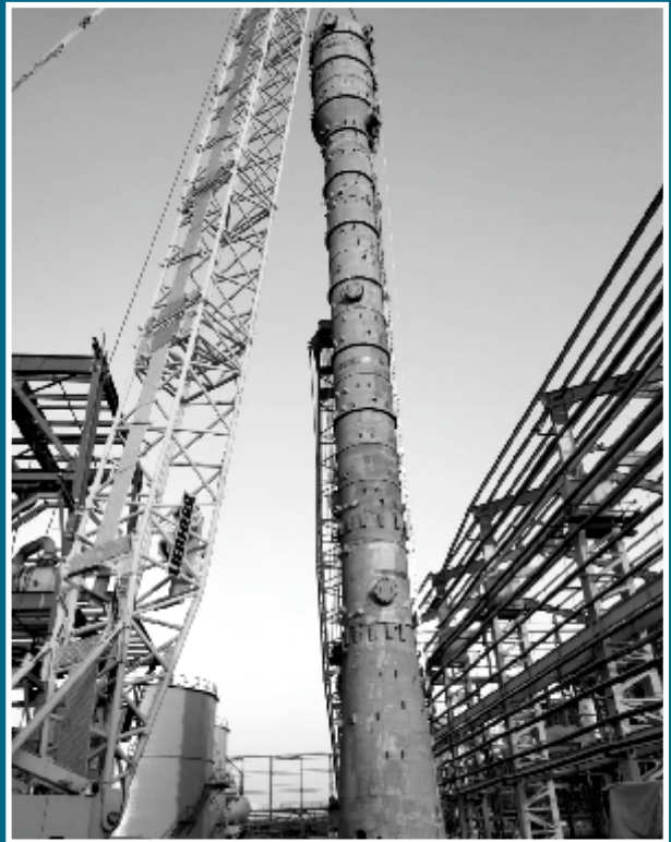
Single Stage Sour Water Stripper Column Erection, 94MT, 44m long & 2.4m dia at IOCL Haldia BS-VI Project
