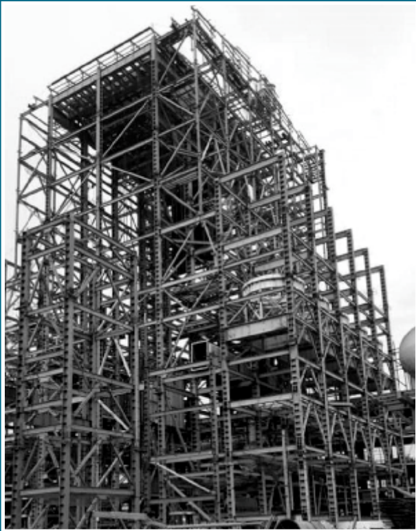
Erection, Testing & Commissioning of Boiler and it Auxilliaries for 2 X 800 MW Ramagundam Project of NTPC
