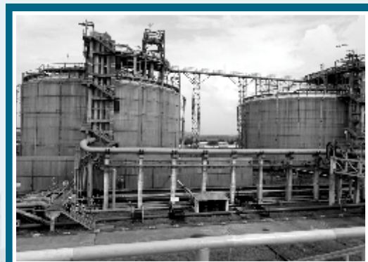
Cryogenic LPG Storage Tank at BPCL Uran
