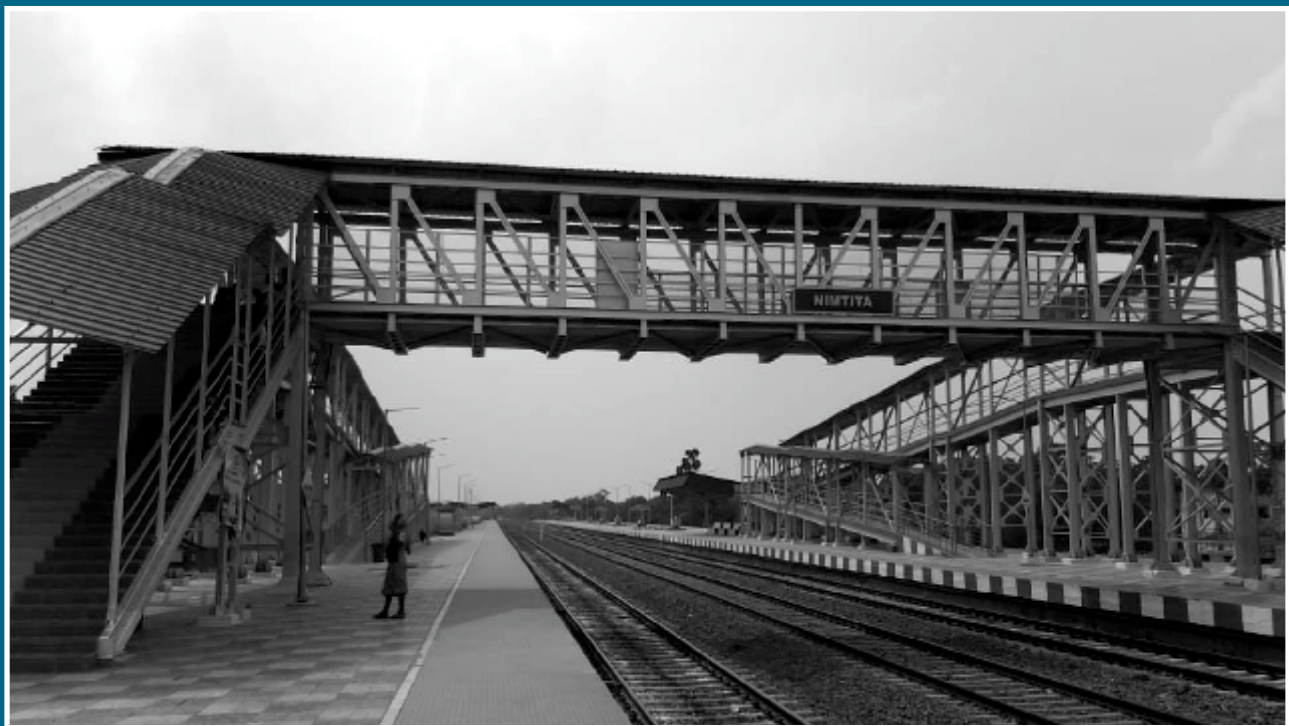
Laying of 19 KM Railway Track along with all the associated work like Platform , FOB , Building etc. in the section from Nimitita to Sujnipara for Eastern Railway
