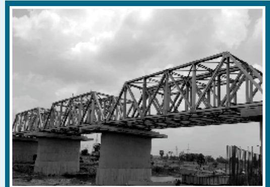
Civil and Structural work of railway bridge over Uthala river at Raghunathpur for RITES
