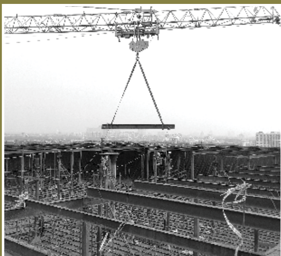
Renewing of 9.0 MG Capacity Century Old Over Head Balancing Steel Reservoir (Tallah Tank) for Kolkata Municipal Corporation
