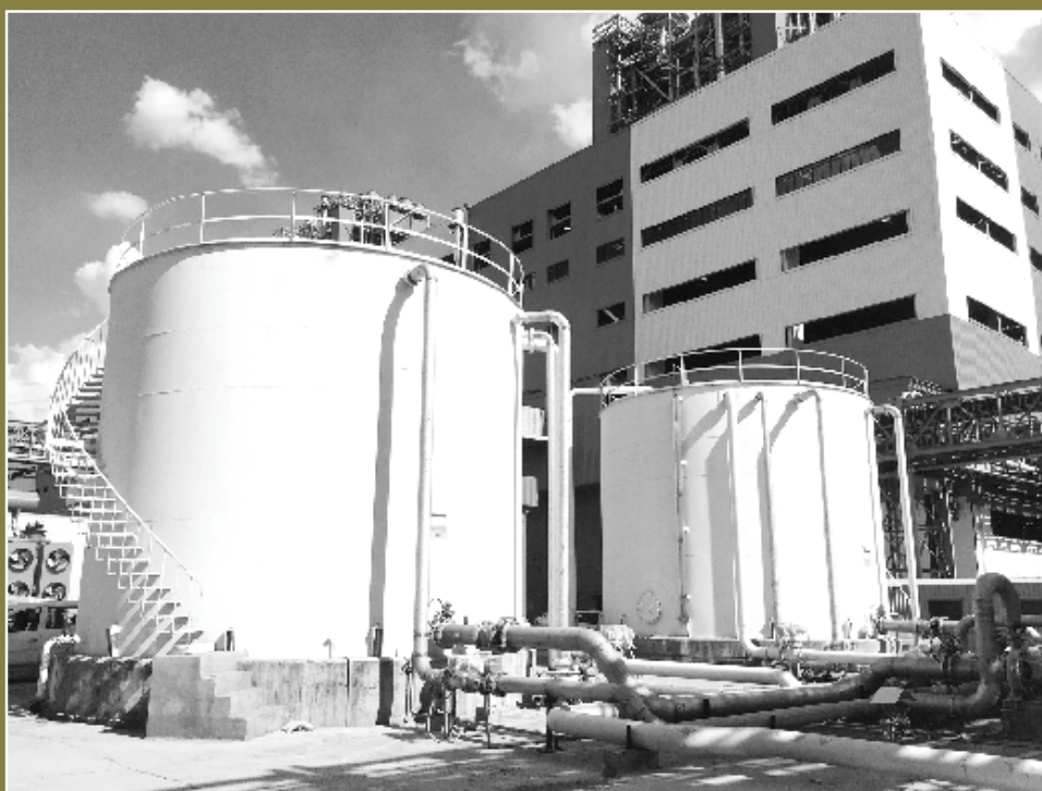
Station Piping Package for Solapur Super Thermal Power Project (2X660 MW), NTPC on Turnkey Basis
