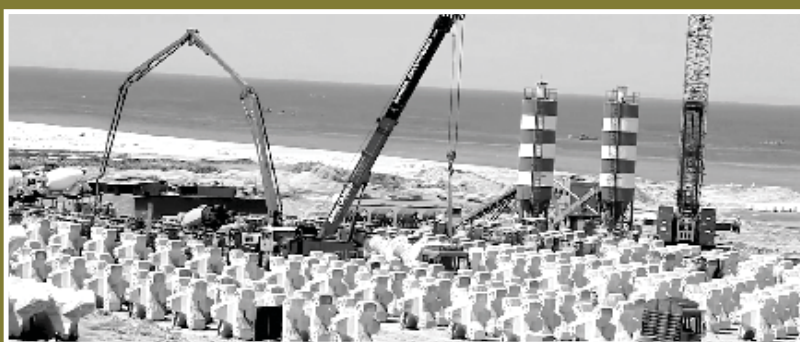
Casting and Staking of Accoropodes-II for break water development of Vizhinjam Port at Kerala for Adani Group
