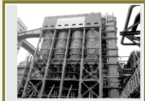
Coal Bunker for 2 X 500 MW Units at Sagardighi STPP of West Bengal Power Development Corpn. Ltd.
