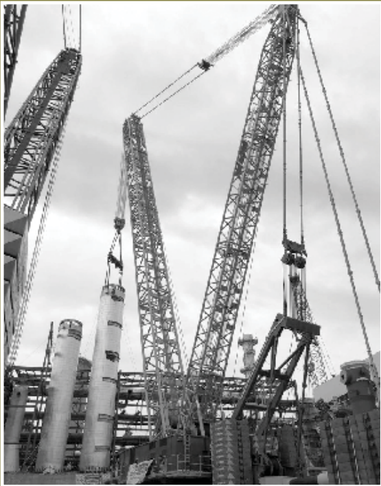
CO 2 ADSORBER column 51 mtr height and 550 MT weight being erected with 1600 MT cap main crane and 600 MT trailing crane at RFCL Ramagundam
