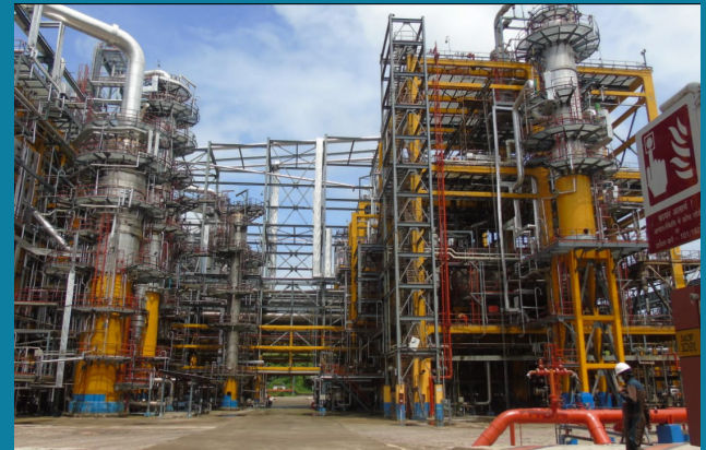
Mechanical Works for Offsites-Refinery Area for Integrated Refinery Expansion Project (IREP) at Kochi, Kerala for BPCL
