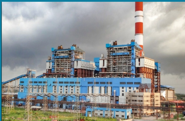
Civil, Structural, Architectural Work Works for Power Block Unit No. 2 (Package-B) comprising of Plant Area Grading and Levelling, Boundary Wall, Main Power House Building (Unit No. 2), auxillary buildings including CW Pump House, Forebayand CW Duct at Andal, West Bengal for BHEL
