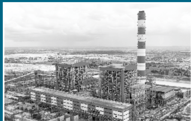
Main Boiler and its Auxiliaries, Piping, Equipment, Bunker & Allied work at NTPC Darlipali 2x800 MW STPP for BHEL
