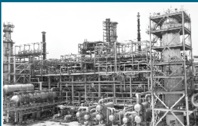
DHT Unit at Bharat Petroleum Corpn. Ltd. Mahul
