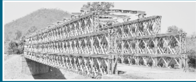
Bailey Type Unit Bridges at different locations in Rayagada, Odisha for Government of Odisha
