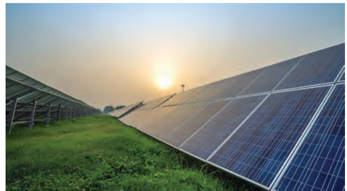
Through 26 MW+ in-house solar power installations, BHEL achieved considerable carbon footprint avoidance
