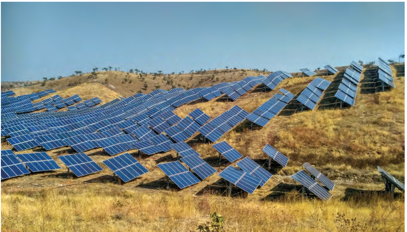
50 MW ground mounted SPV plant commissioned by BHEL at NTPC, Mandsaur
