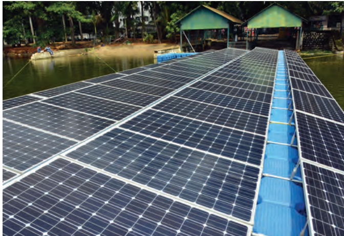
Floating solar plant commissioned by BHEL at Ulsoor lake, Bengaluru
