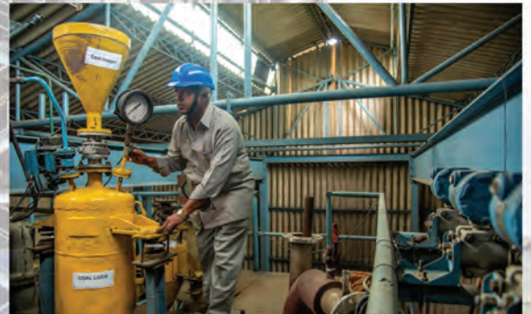
Coal Feeding System
