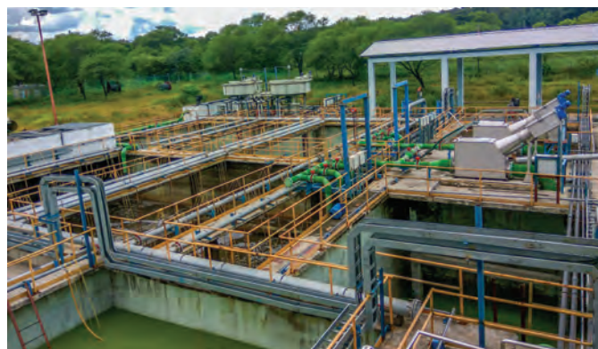
Membrane bio-reactor (MBR) based sewage treatment plant (STP) commissioned by BHEL in Hyderabad
