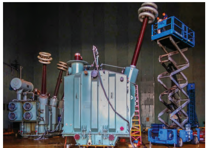
High Voltage test lab at BHEL, Bhopal
