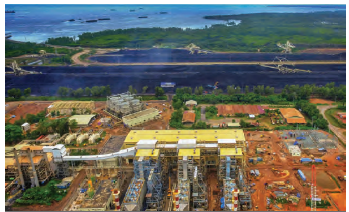
Aerial view of three units of 3x18 MW PT CKP project at Indonesia, commissioned by BHEL
