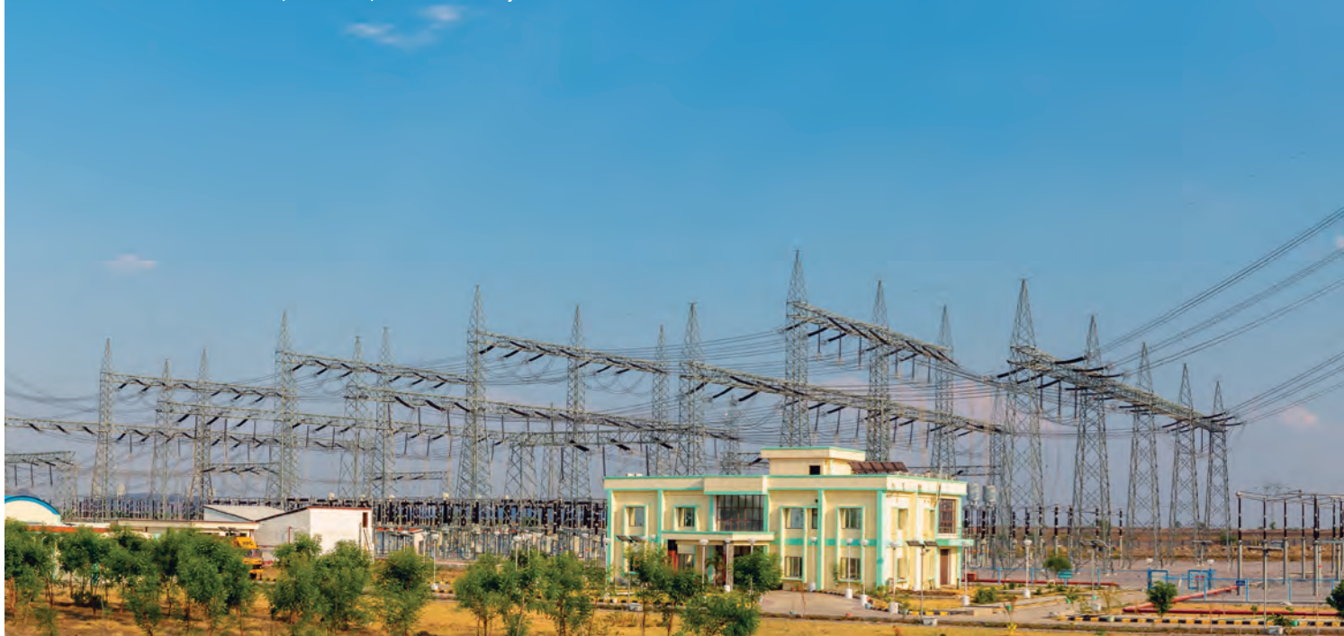
765/400 kV substation at Raichur, Karnataka, commissioned by BHEL
