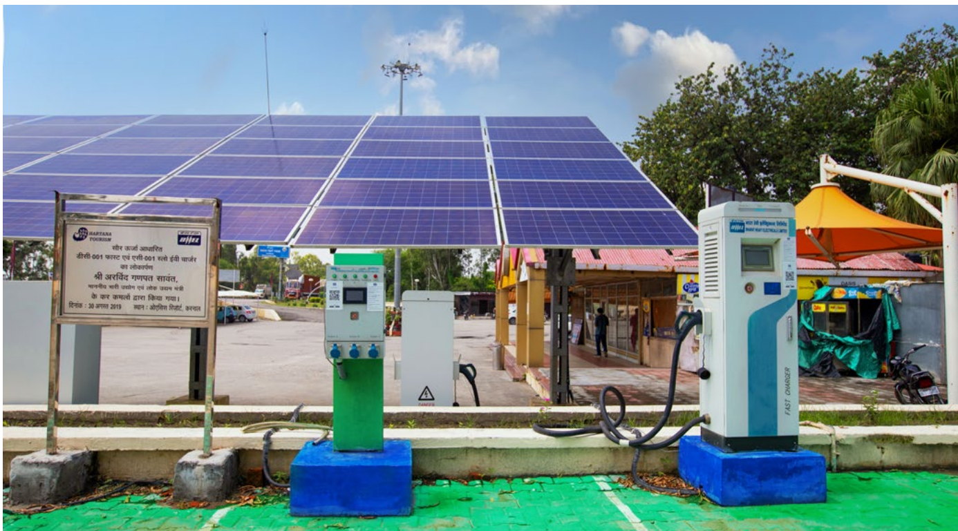
The Delhi-Chandigarh Highway has become the first e-vehicle friendly highway in the country, with a network of Solar-based Electric Vehicle Charging stations (SEVCS) set up by BHEL under the FAME-1 scheme of the Ministry of Heavy Industries
