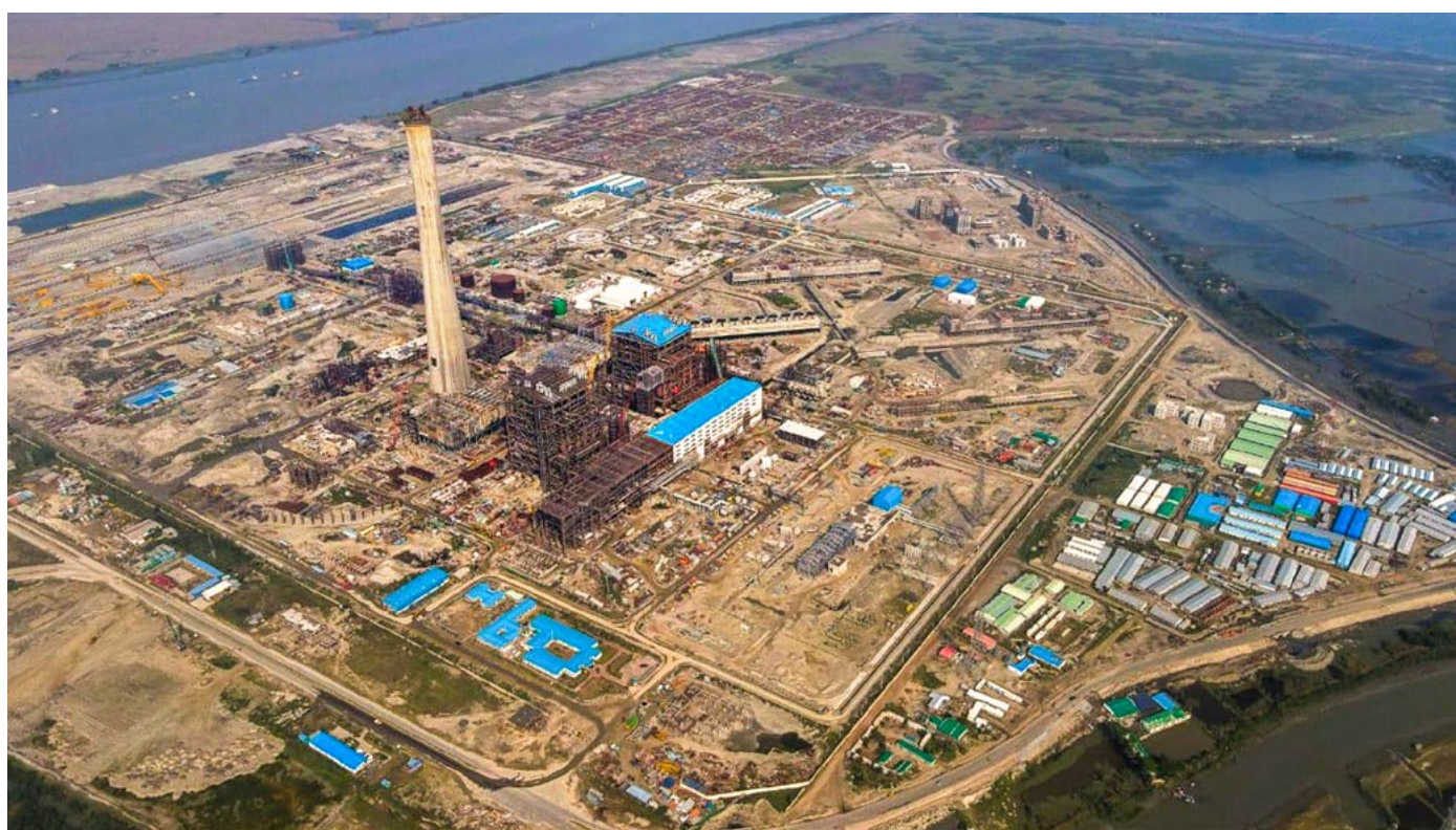
2x660 MW Maitree Supercritical Power Project being executed by BHEL in Bangladesh
