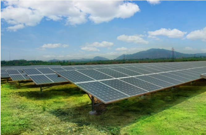
5MW in-house Solar PV installation at BAP, Ranipet for captive power generation
