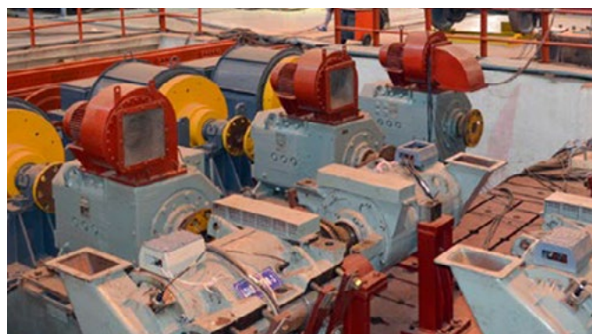
Centre for Electric Transportation (CET) at BHEL Bhopal
