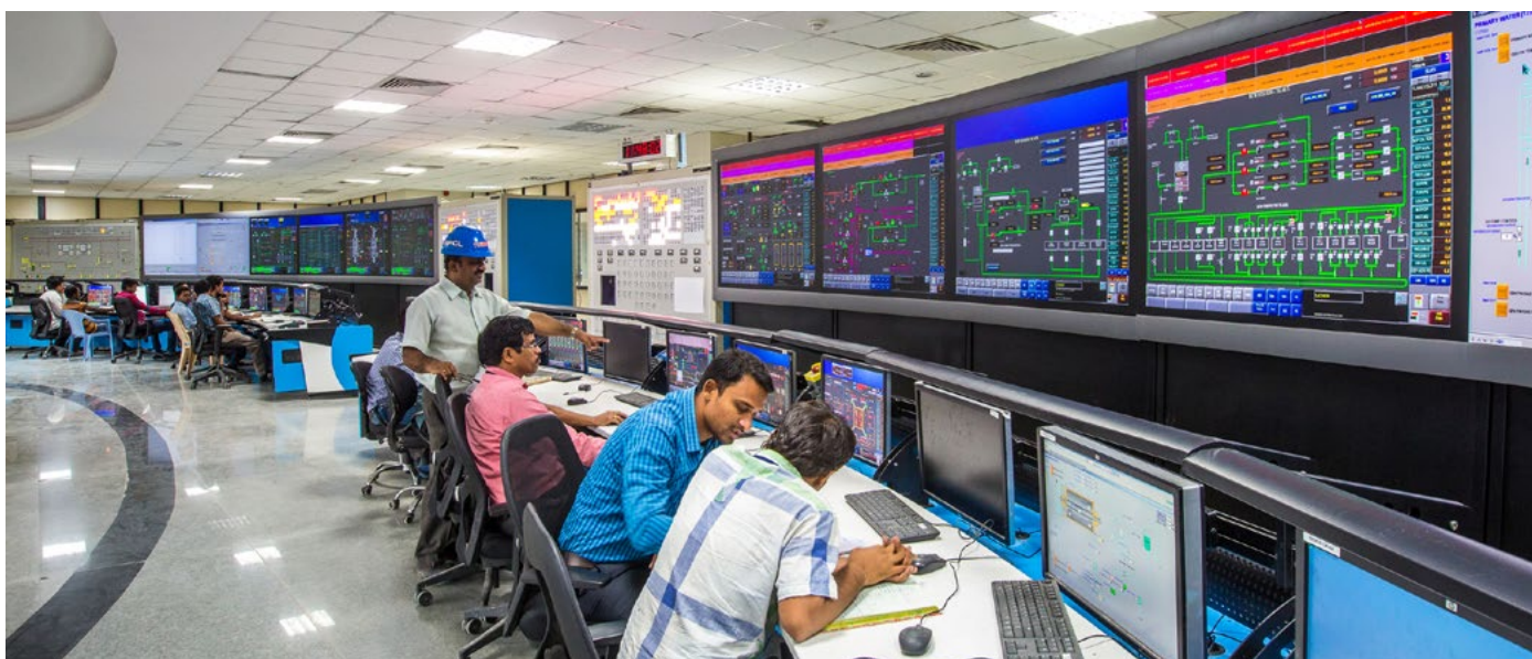
State-of-the-art control centres for power plant operations have been set up at all its commissioned units by BHEL
