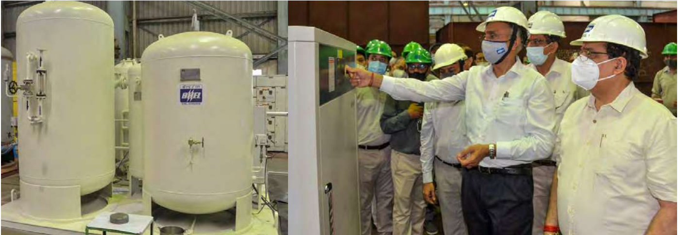
Medical Oxygen Plant at BHEL, Haridwar
