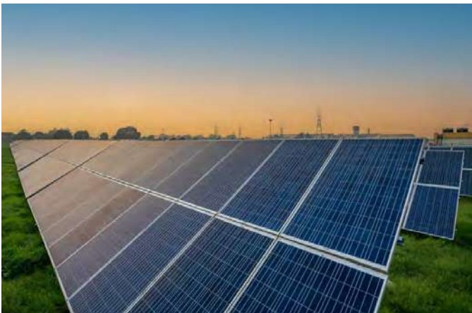
5MW in-house Solar PV installation at BHEL Haridwar for captive power generation
