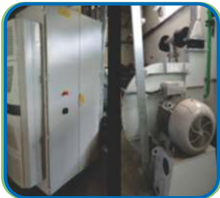
Upgraded Conditioned Air Handling Unit (CAHU) for High Altitude Simulation
