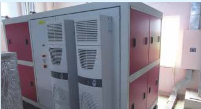
◀ Conditioned Air Handling Unit ▶
