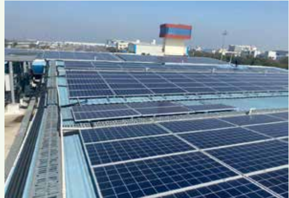
Solar Energy Power System at iCAT- Manesar
