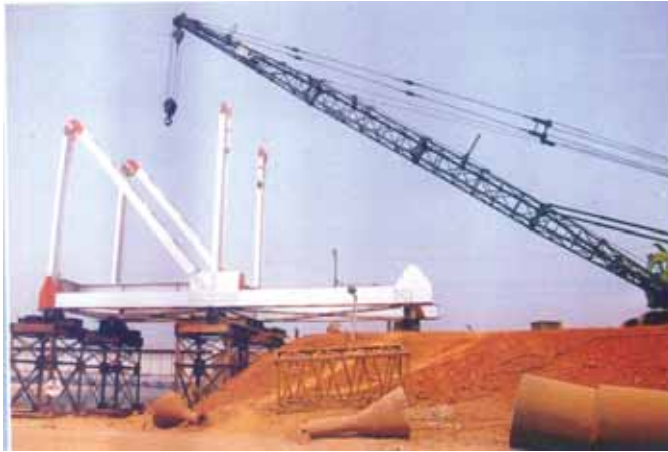
Bridge over Mahanadi river at Cuttack under construction by Braithwaite Burn & Jessop Construction Co. Ltd.
