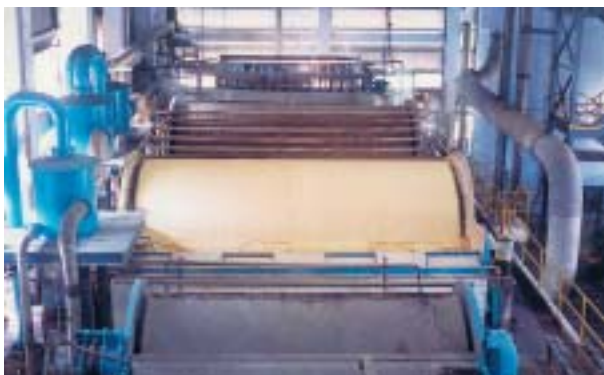
CMP Washing Plant of HPC
