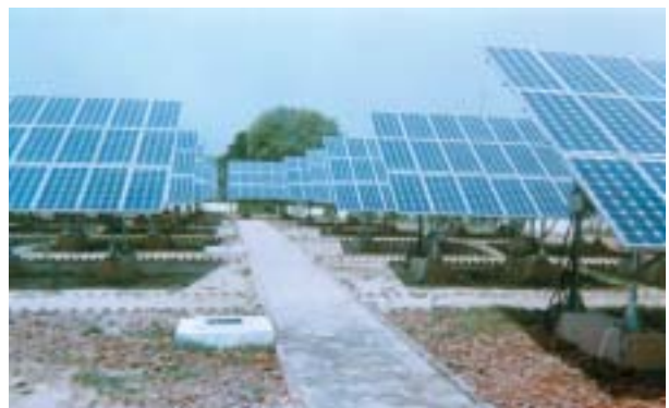
SPV Grid Interactive Power Plant (50 KWp) for boosting grid tail-end voltage manufactured by REIL
