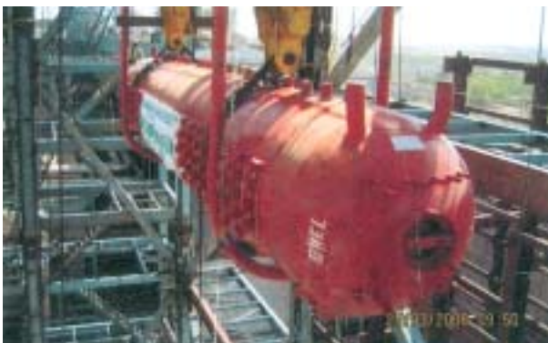
Erection, Testing and Commissioning of Boiler Main (130 MT at Elevation 56M) at 1x210 MW Mejia TPS (Unit-IV) of DVC by B&R
