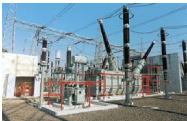
400 KV, 50 MVAR Controlled Shunt Reactor at Itarsi Switching Station, supplied by BHEL
