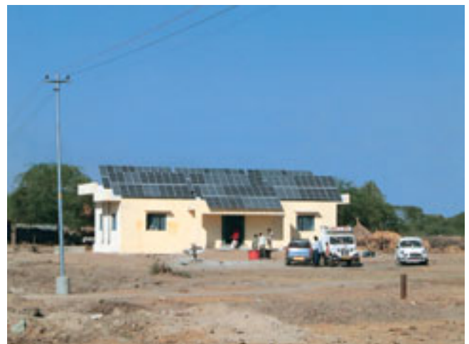
A view of Solar Power Plant installed by REIL at village Kheri in Bhilwara district, Rajasthan
