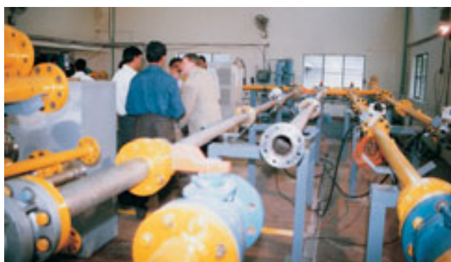
20 Bar Close Loop Air Test facility, being inspected by experts from Netherlands, at FCRI
