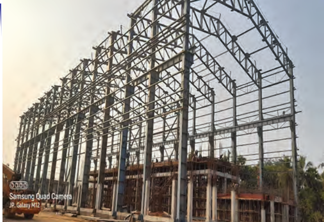
Rare Earth Permanent Magnet (REPM) Plant at BARC, Visakhapatnam
