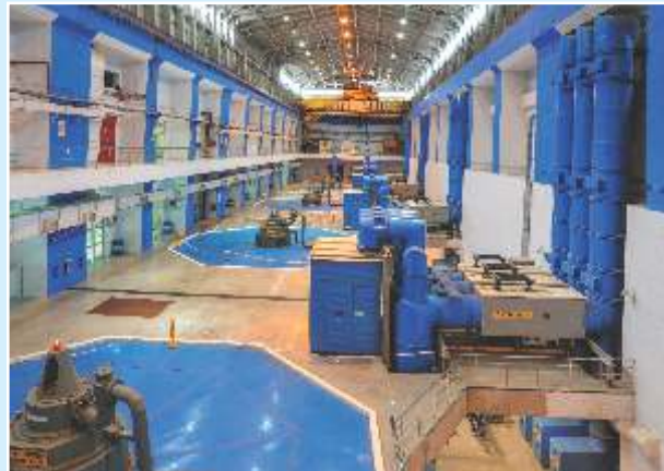
800-MW Koldam Hydro Power Plant
